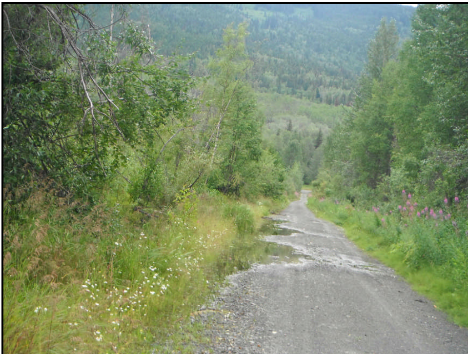
Photo 3: Looking east on 26-Mile FSR, road flooding caused by beaver dams (August 10, 2012).
